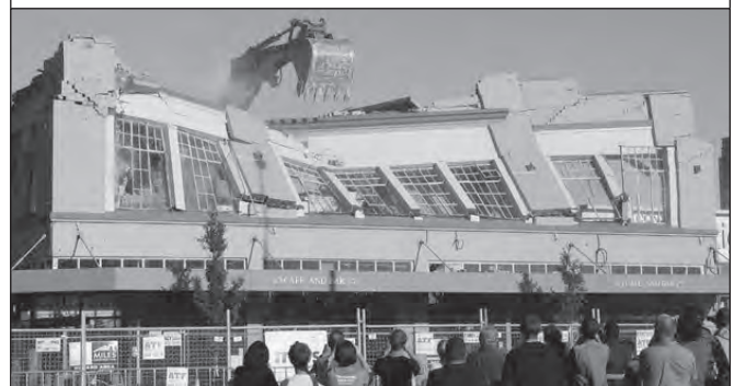
A crowd watches as the Lone Star Restaurant in Manchester Street is demolished
