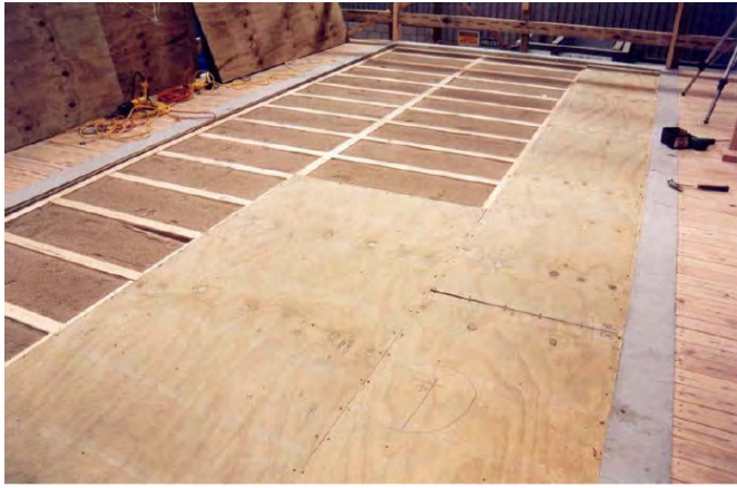
Figure 3. View of plywood flooring over 70x45mm battens laid on the flat with sand infill.
