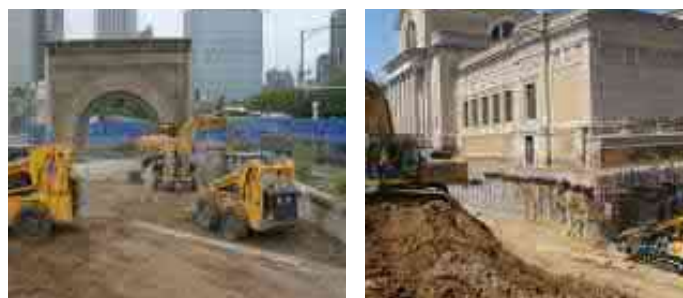
Figure 11. (Left) Site grading adjacent Sullivan Arch which lies adjacent to the Modern Wing addition at the Art Institute of Chicago. (Right) Construction works adjacent the Saint Louis Art Museum, Saint Louis, Missouri, construction underway for expansion, 2010 (5)
