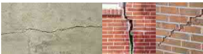
Figure 13. Examples of cosmetic vibrational construction damage (left) and (right) and structural vibrational damage (3)
