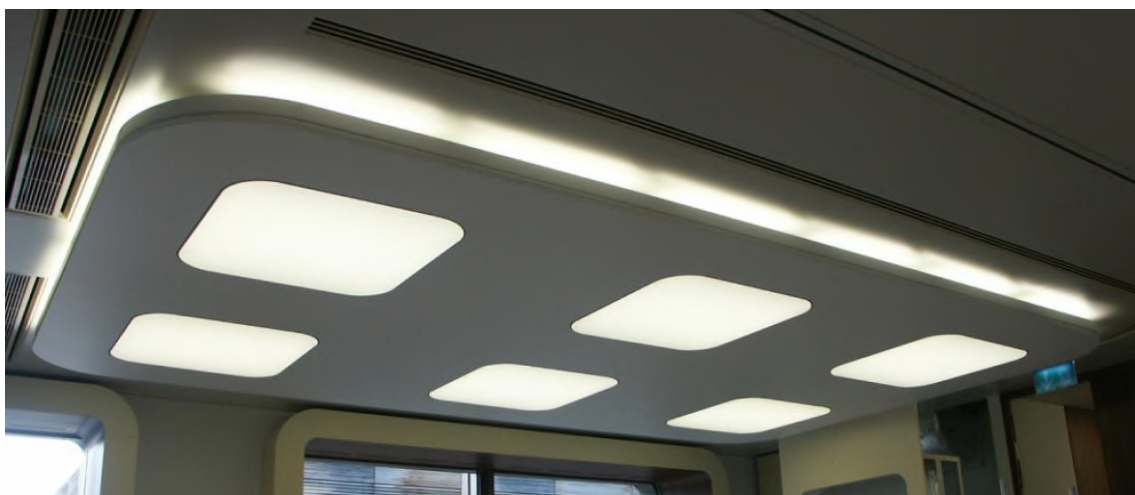
Figure 5: Lighting system/sound absorbing ceiling in an office.
