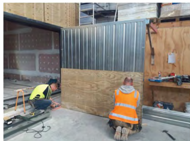
Figure 7 – Transmission loss opening with collar and plug
